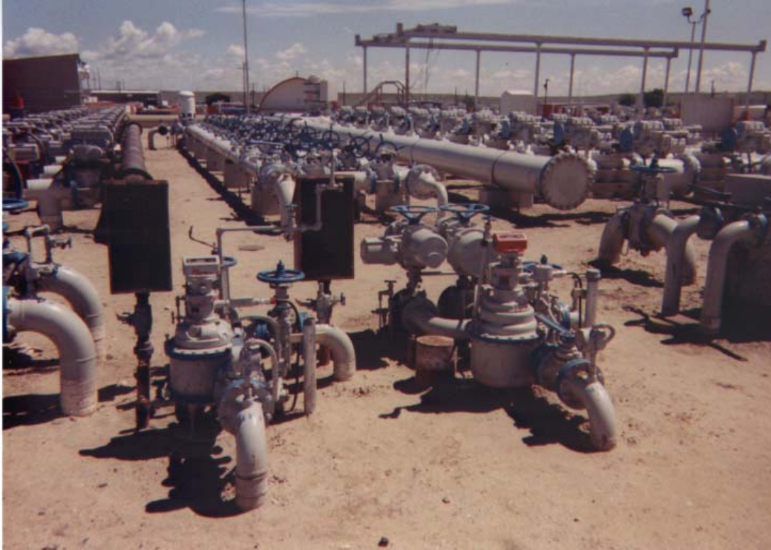
Casper Station Yard Valves
